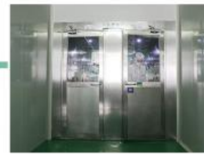
7. Go through the air shower room
