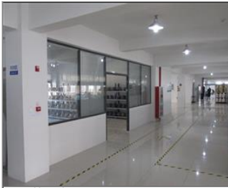
Photo of fire safety equipment Fire equipments.JPG
