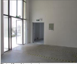
Photo of fire safety equipment Emergency exits.JPG
