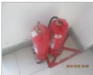
Photo of fire safety equipment Fire extinguishers.JPG
