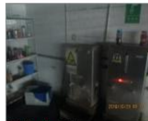
Photo of the sanitary facilities Potable water.JPG
