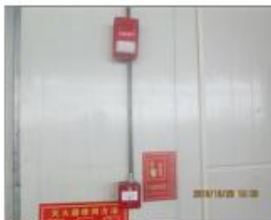
Photo of fire safety equipment Fire alarm.JPG
